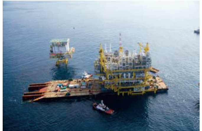
The Intermac 650 after modifications ready to perform it's first topside floatover in Asia Pacific.
